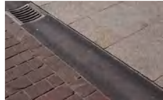
Kolk in betonnen molgoot
